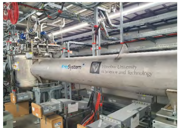
Figure 1. Cryogenic Distribution System designed by WUST, now under commissioning at ESS, Lund, Sweden.
