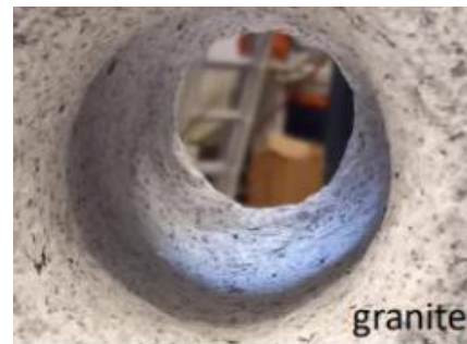
Thermally spalled borehole
