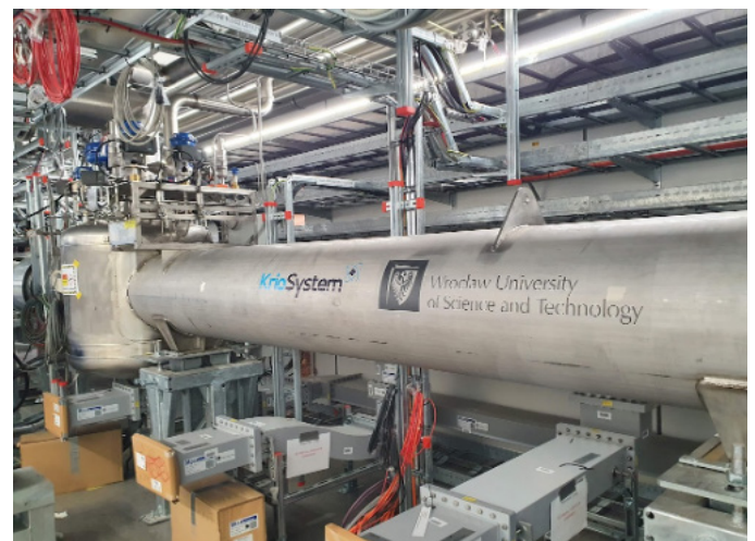
Figure 1. Cryogenic Distribution System designed by WUST, now under commissioning at ESS, Lund, Sweden.
